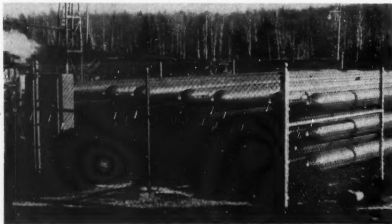
The "Cascade" oxygen supply unit which supplies oxygen to the Erie Mining Company's JPM-1 Jet-Piercing machine at Aurora. Gaseous oxygen is stored here at high pressure and released automatically at lower pressures as needed.
